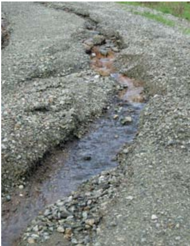
Figure 55. Erosion from driveway in Jordan/Alder Watershed.
